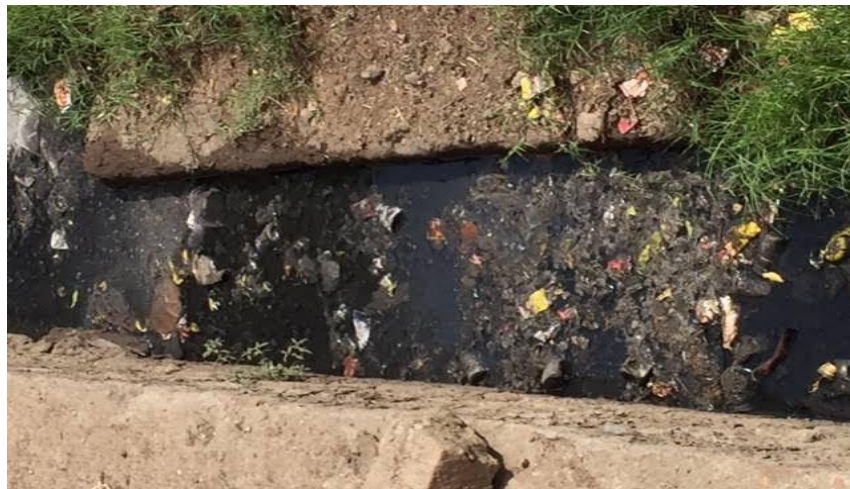
Fig.3: Domestic wastewater sewer of Shastri Nagar
