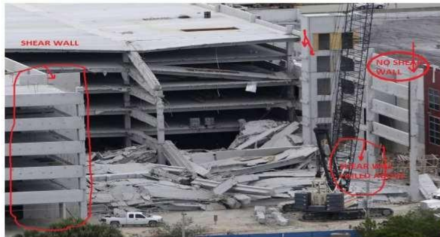
Figure 2.11 Failure Due to Shear Wall [23]
