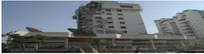
Figure1: Failure of R.C. Building with floating columns
