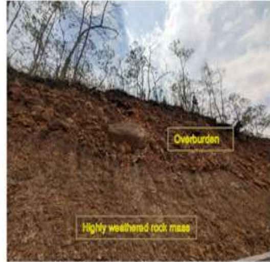
Figure 3: Unstable zone at the top of slope between Ch. 12+850 km and Ch. 12+950 km.
