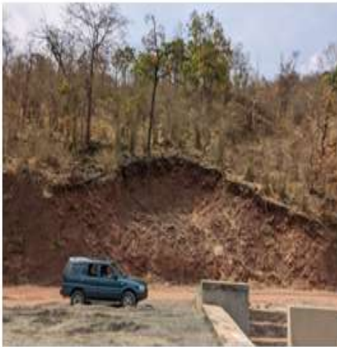
Figure 4: Slide Near to Bridge No. 27
