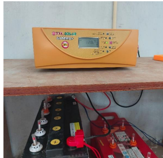
Fig 5 Inverter And Battery
