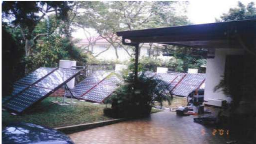
Fig.(4): Multi Solar System
