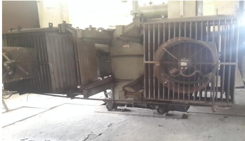
Fig.1. Transformer cooling fans
